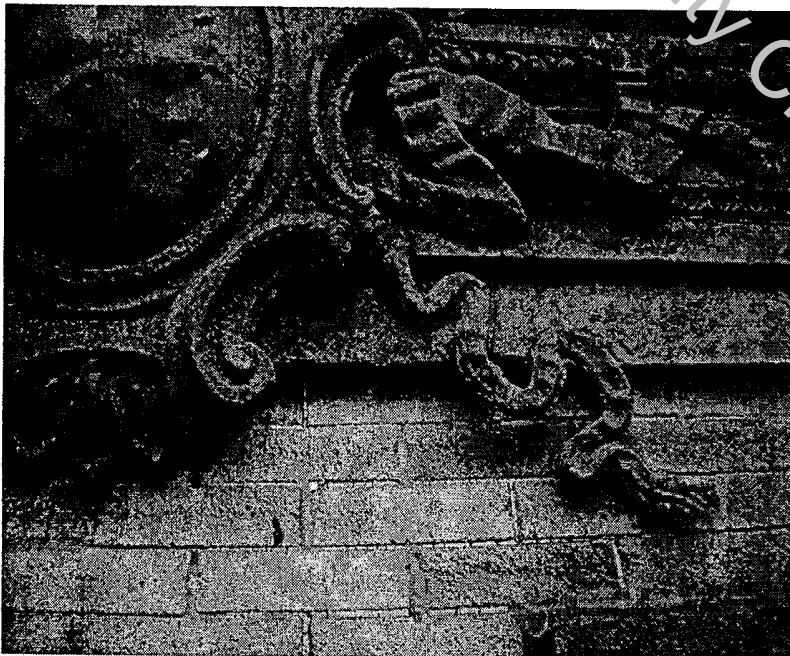
Figure 9 - Sheet metal medallion and ribbons on west facade. Numerous supplemental fasteners have been previously added to the various components which comprise the medallions. Loose components were removed at the time of our inspection.
